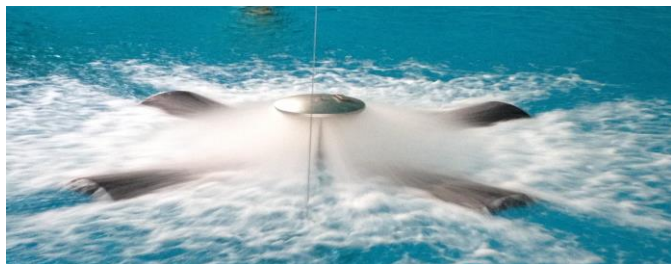
Aeration equipment used to remove THM's
